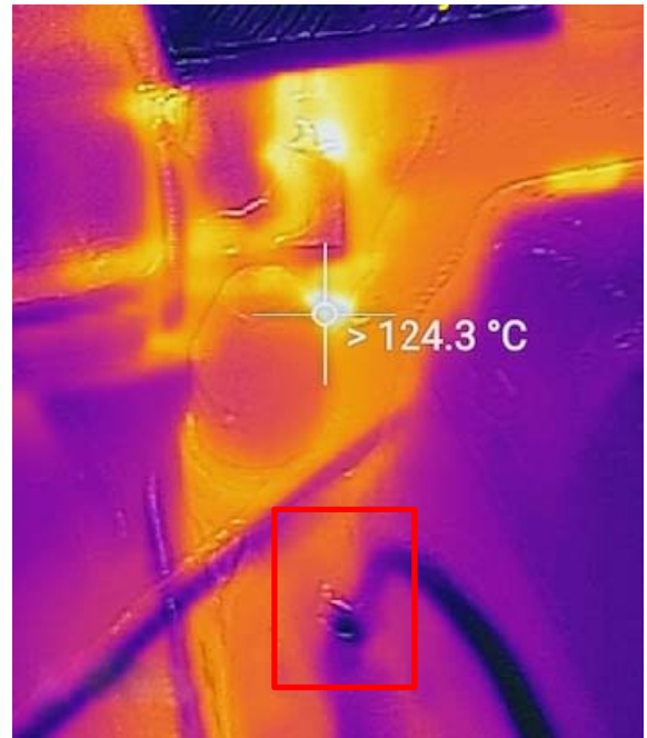
Figure 10. Hotspot close to cylinder no.17's fuel return circuit connection.
